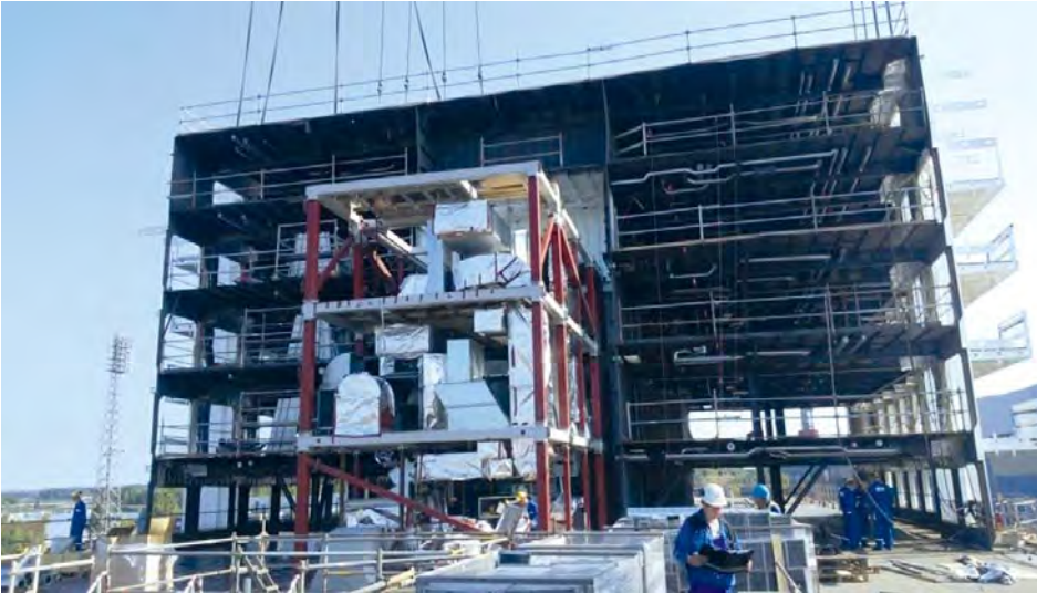
Figure 1. AC room module installed on board the ship in the dry dock, and the grand block is lifted over it
