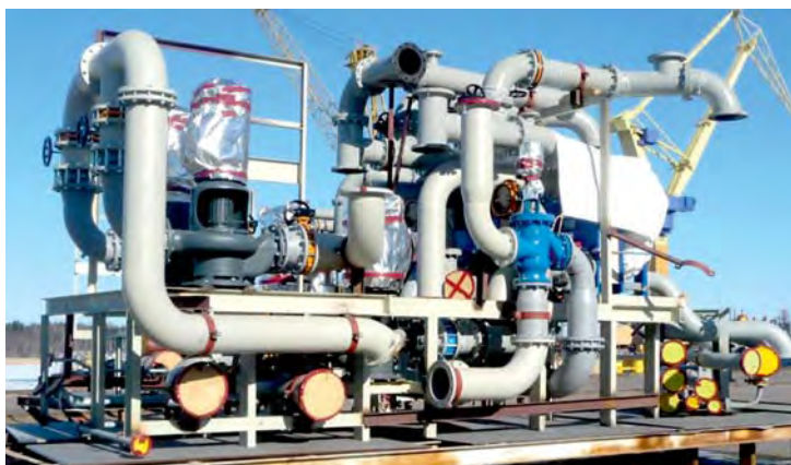
Figure 6. One of four engine room modules
